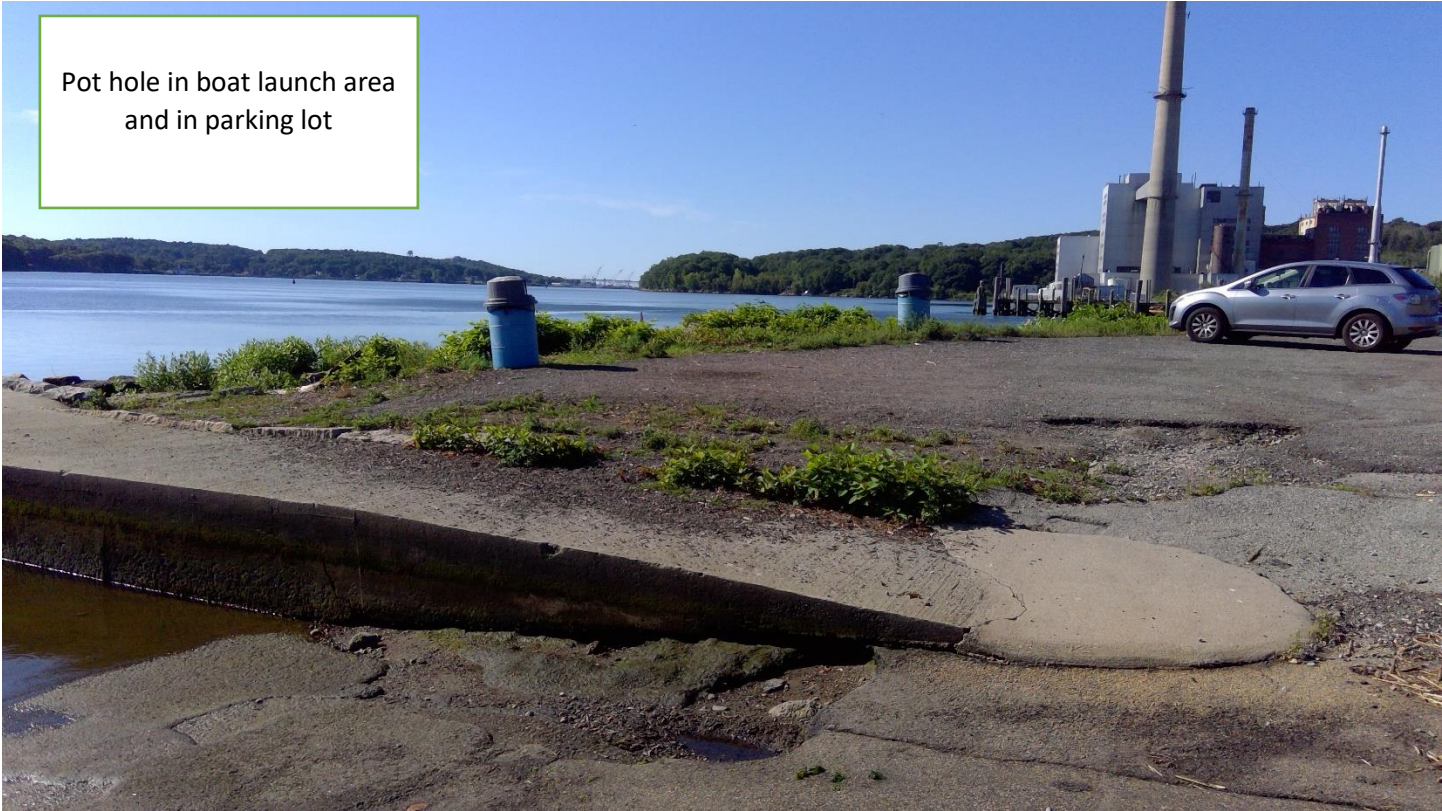
Pot hole in parking area
