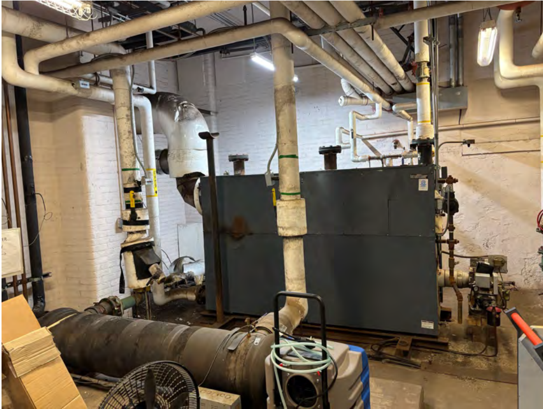
Existing Boiler: Age unknown (estimated 1956-1966)
