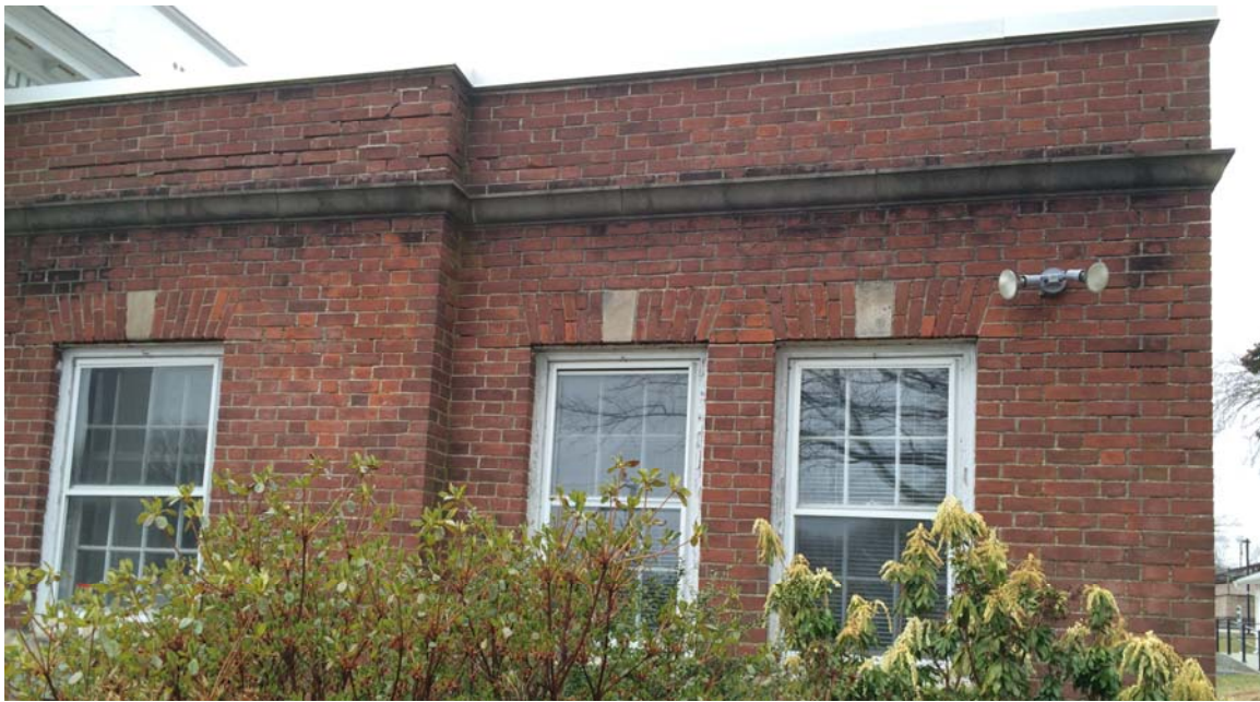
Figure 1: East Face, North End, General Conditions Include: Cracking, Mortar Washout, Spalling, Lintel Displacement
