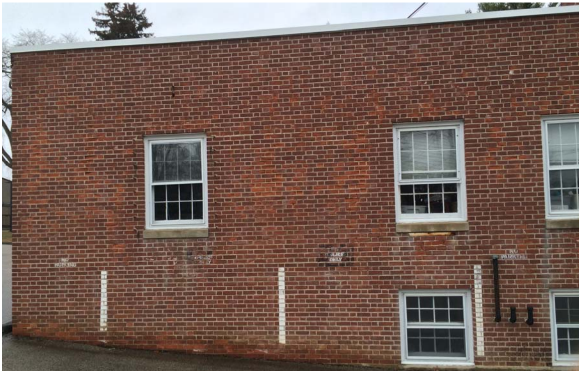
Figure 2: South Face, West End, Severe Spalling
