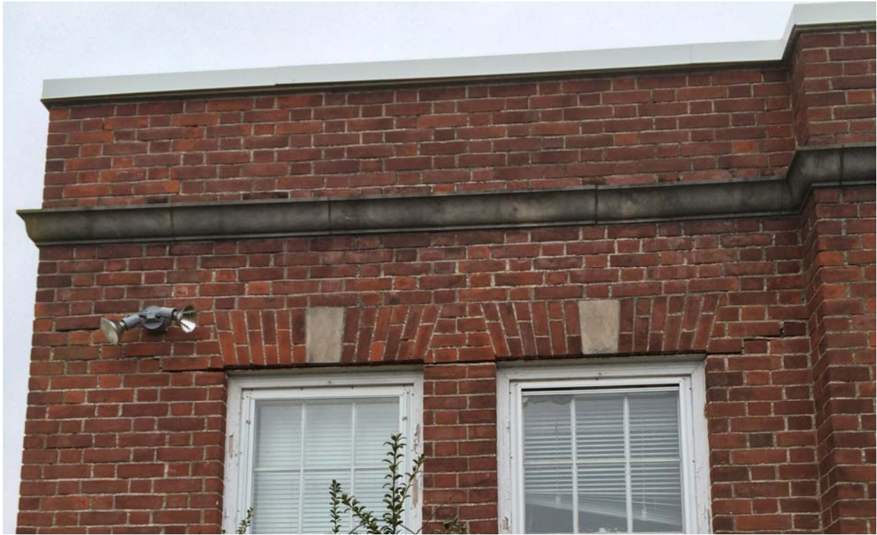
Figure 3: East Face, South End, Severe Lintel Displacement
